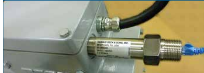
INSTALLED BECK MODBUS TCP ADAPTER
