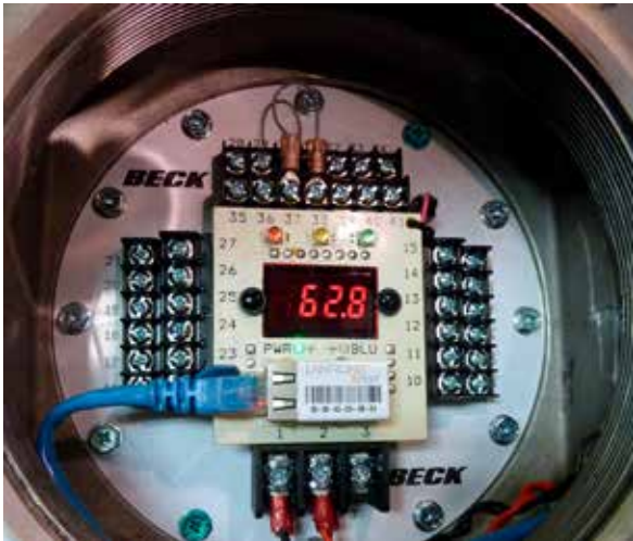
BECK MODBUS TCP DEVICE INSTALLED ON THE TERMINAL BLOCK
