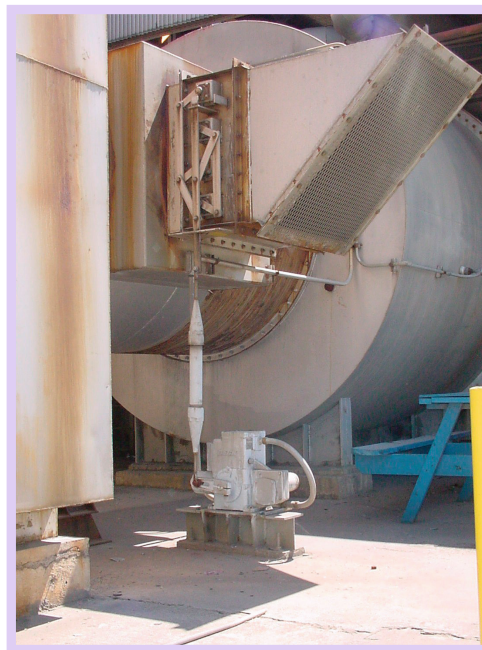
i.e. Beck rotary 11-409 [Melt Shop Fume Control Tempering Air Damper]
