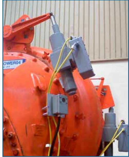
42-109 oriented skyward on an inlet guide vane blower
