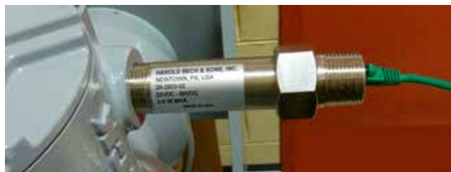
INSTALLED BECK MODBUS TCP ADAPTER
