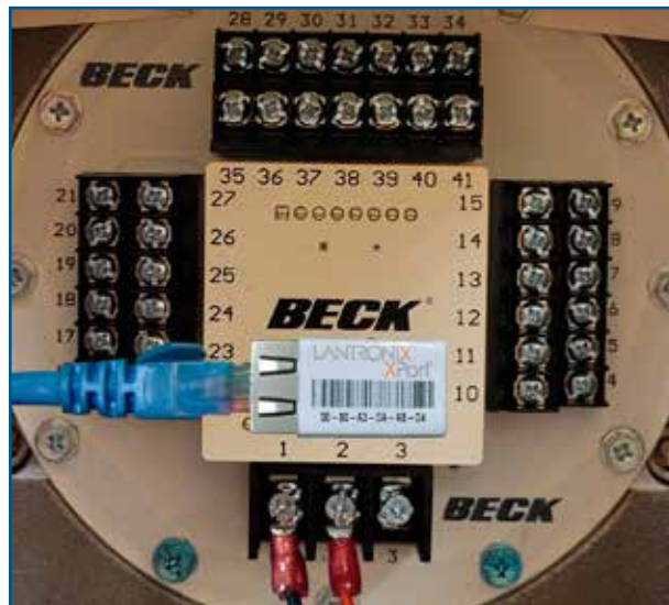
BECK MODBUS TCP DEVICE INSTALLED ON THE TERMINAL BLOCK
